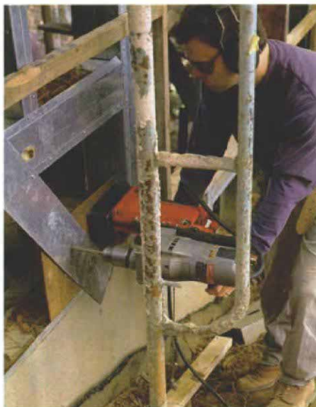
This drill is self-supporting. An electromagnetic drill press clamps onto a workpiece. Here the author drills \frac{1}{2} -in. holes in a \frac{1}{4} -in. steel hold-down and a 16-ga. diagonal strap.
