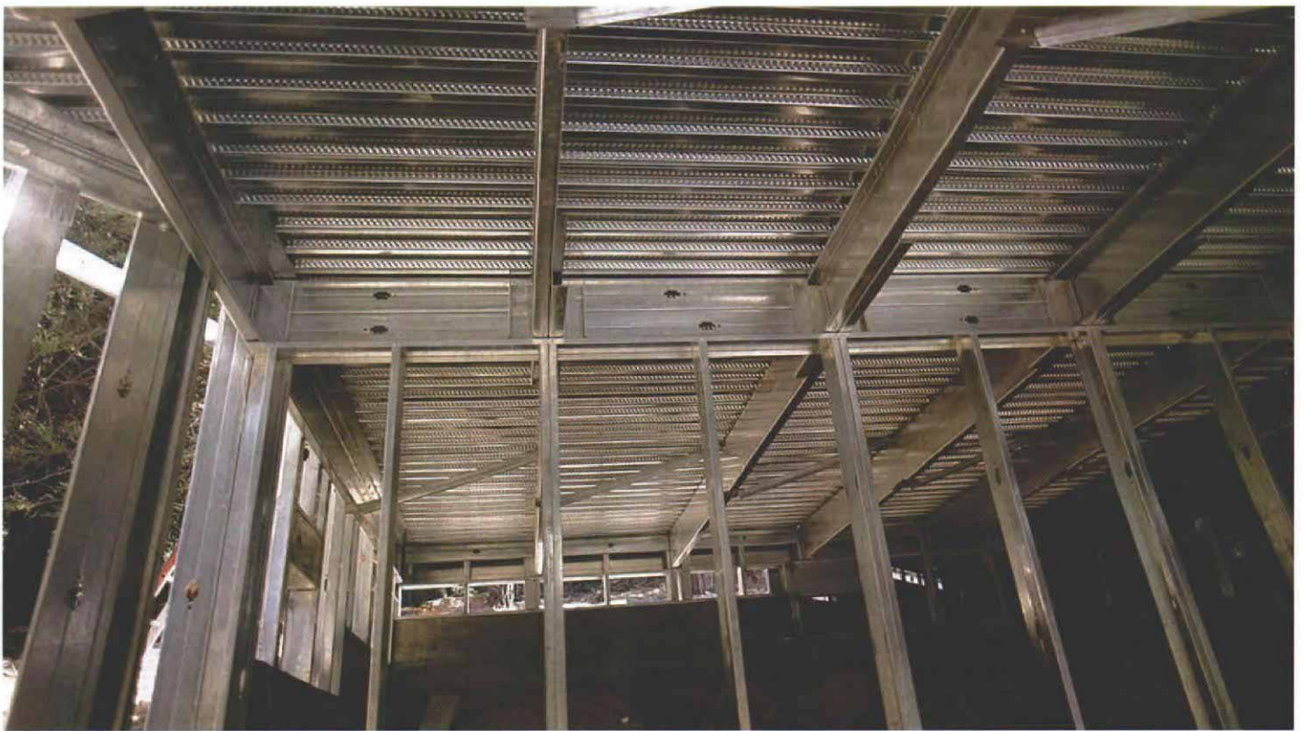
The view from the crawlspace. Joists at 4 ft. o. c. carry the corrugated metal deck of the main floor. Each joist is carried by a pair of studs. At the pony wall in the background, web stiffeners midway between the joists car-
